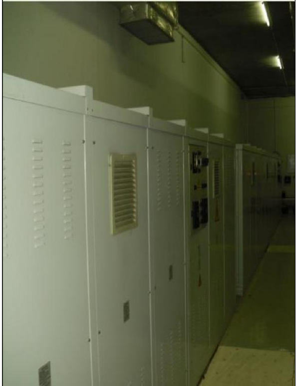
Salle MT-Batteries HTA
