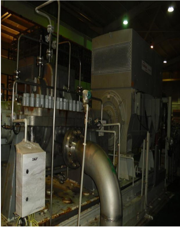
OSMOSE (Pompe HP)
