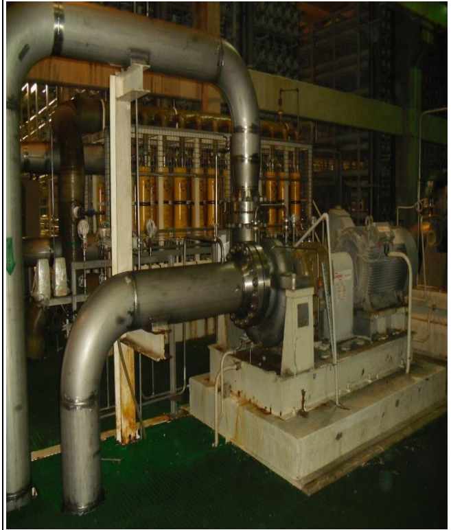
OSMOSE (Pompe Booster)
