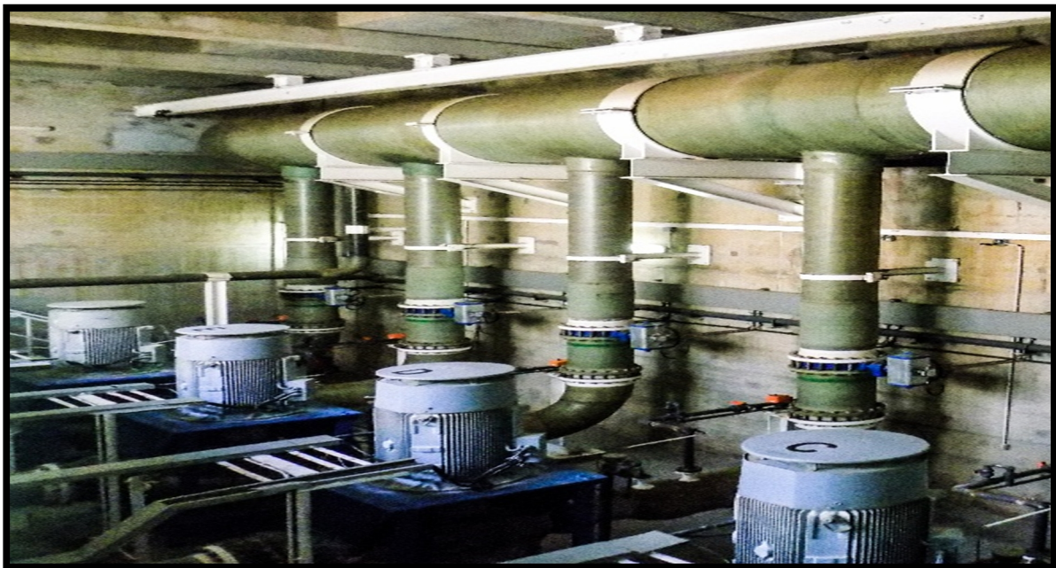
Figure 19: Station pompages eau de mer
